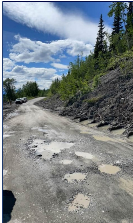
Figure 4-12. McCarthy Road Conditions near MP 58
